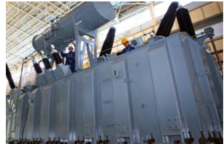
Wind power transformers
